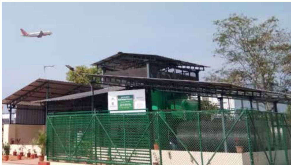
500 kg/day food waste biogas plant installed at Trivandrum International airport
