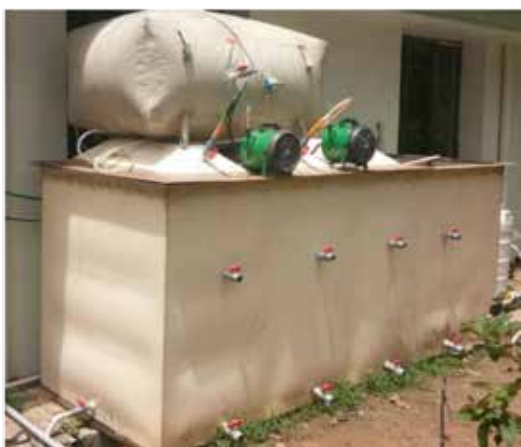
NOWA unit (2000L/day) installed in NIIST campus recovering biogas and reuse quality water from high strength wastewater discharged from NIIST canteen
